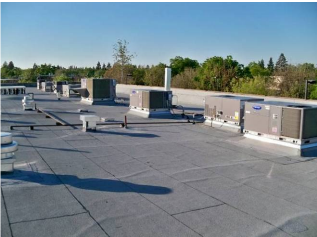
5. View of HVAC package units on Building 1445 roof (typical of most buildings).
