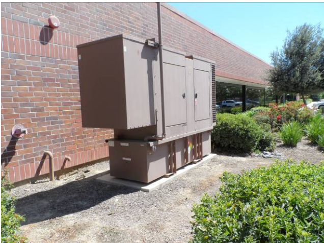
6. View southeast of standby generator and diesel fuel "belly" tank at northwest corner of Building 1445.
