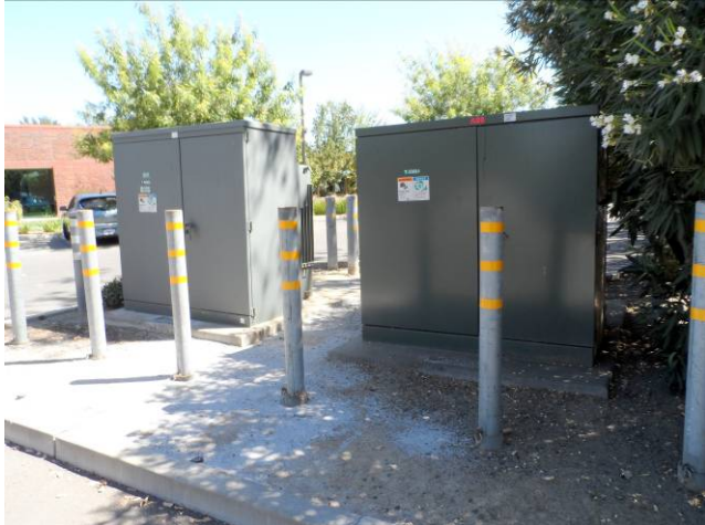
19. View southeast of PG&E transformers in central portion of subject property (typical).
