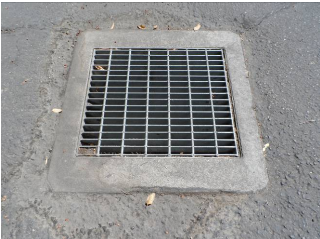
18. View of stormwater drain in interior drive (typical throughout drives and parking areas).
