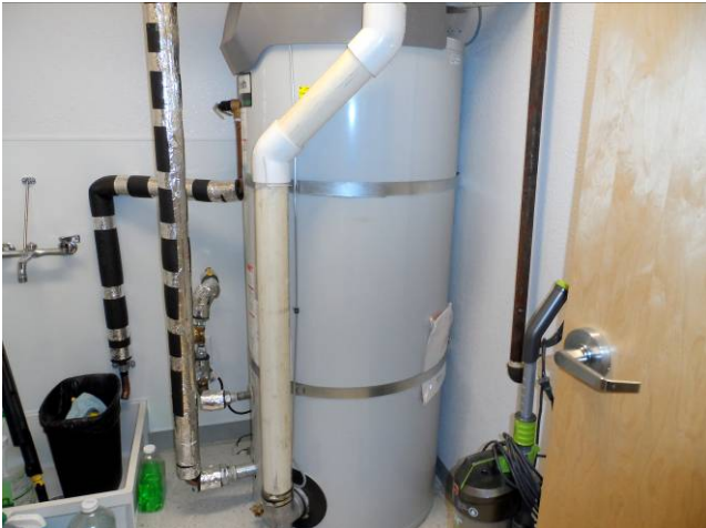
15. View of natural gas-fueled water heater unit in Building 1940 utility room.
